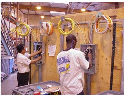
Left: Panels with homeruns for apartment units.
